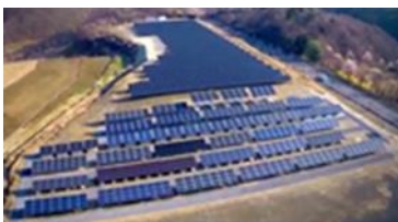
Solar photovoltaic power plant (Sukagawa and Tamagawa Village, Ishikawa, Fukushima Prefecture)
