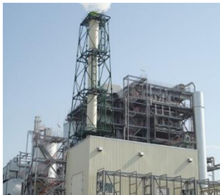
Biomass power plant (Kawasaki, Kanagawa Prefecture)
