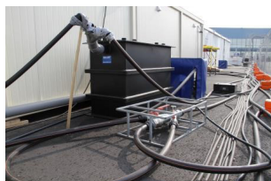
Temporary water supply and drainage system
