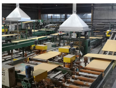
Ventilation hoods over a coating line
